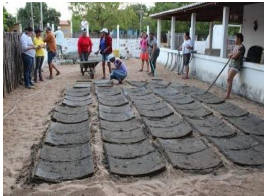
Figure 4. Training and interchange between the local group and CF8 for the construction of fertilized cisterns in Apodi (State of Rio Grande do Norte), 2019.
