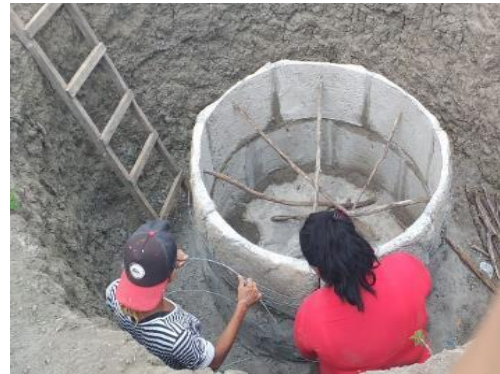
Figure 5. Construction of the reuse filter by women in the Hipólito Settlement in Mossoró (State of Rio Grande do Norte), 2020.
