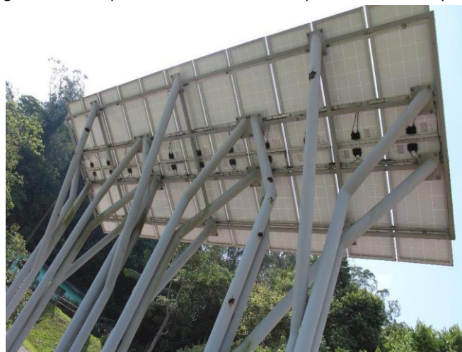
Figure 8 – Lower part of the infrastructure of photovoltaic solar system
