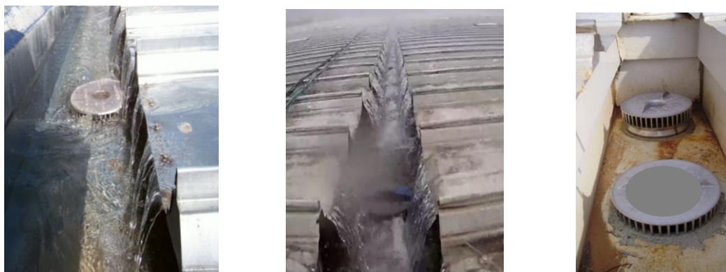
Figure 7 – Section of gutter with rain and semi-submerged and fully submerged outlets (A) in emergency system (B)
