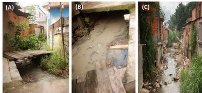
Figure 6 – A. Irregular constructions near the Tributary in Cararu Street. B. Dumping sewage directly into the Tributary in Cararu Street. C. Occupation on the banks of the Popuca stream in the vicinity of Cataguases Avenue.
