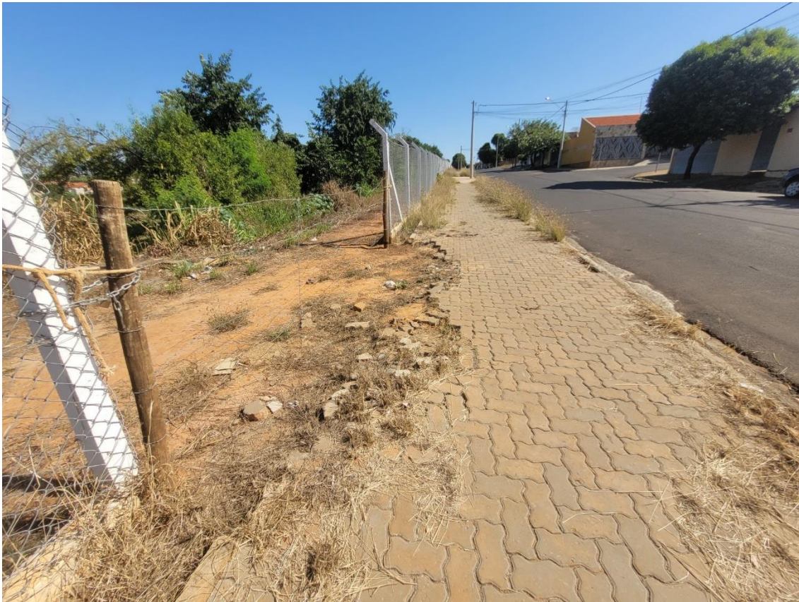
Figure 6 - Wire fencing and padlock, along the deteriorated sidewalk
