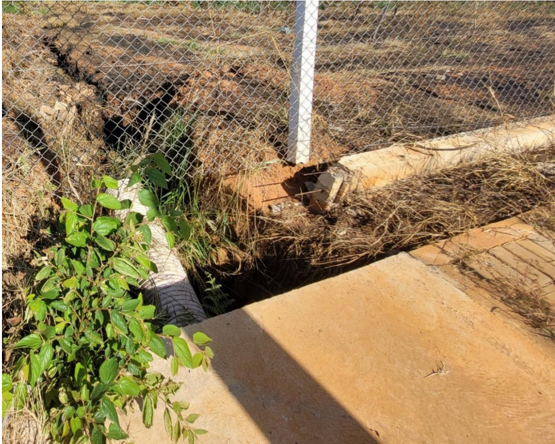
Figure 5 - Scorch marks and erosion mark
