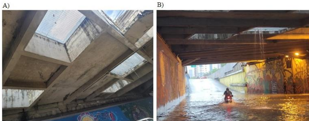
Figure 6 - Detail of the open areas for ventilation and illumination (A) and inside the tunnel during the rainy season (B).
