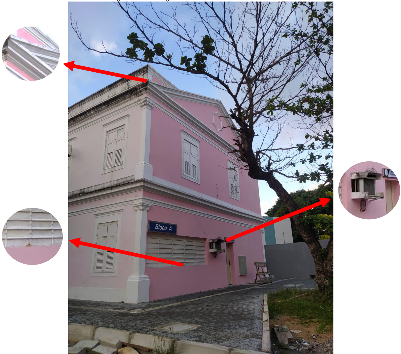
Figure 6 – Pathological manifestations on the South Facade.
