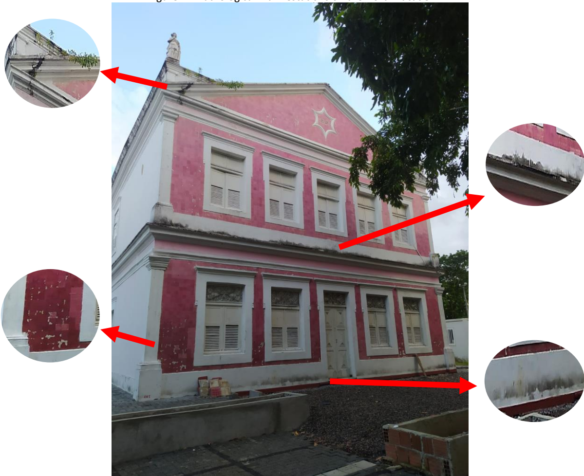
Figure 4 – Pathological manifestations on the North Facade.
