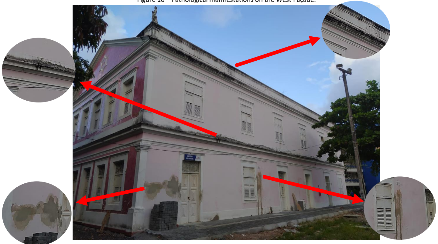
Figure 10 – Pathological manifestations on the West Façade.
