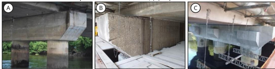
Figure 10 – Process of recovery of the crossbeam. (A) Crossbeam of the bridge without maintenance; (B) Execution of the recovery of the crossbeam block; (C) Repaired structural element
