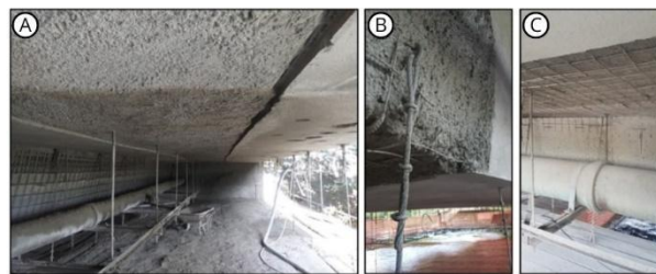
Figure 11 – Deck recovery process of the bridge. (A) Scabbling on the deck; (B) Projected concrete; (C) Installation of reinforcements on the deck
