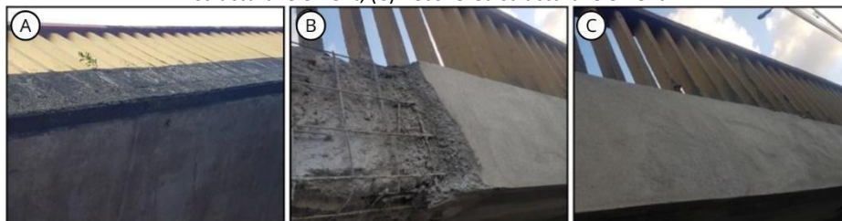
Figure 12 – Walkway slab recovery process. (A) Condition of the walkway slab before recovery; (B) Covering of the structural element; (C) Recovered structural element
