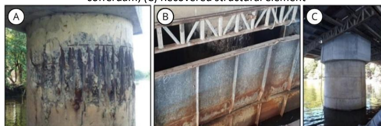
Figure 9 – Caisson Recovery Process. (A) Caisson of the bridge in a deteriorated state; (B) Recovery process inside a cofferdam; (C) Recovered structural element
