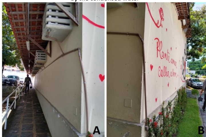
Figure 1: (A) Condensed water collection system of the attached ground floor building; (B) Garden area irrigated by the condensed water
