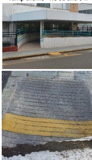
Figure 9: Some problems related to the Curb ramp theme - RC 01 and 04.
