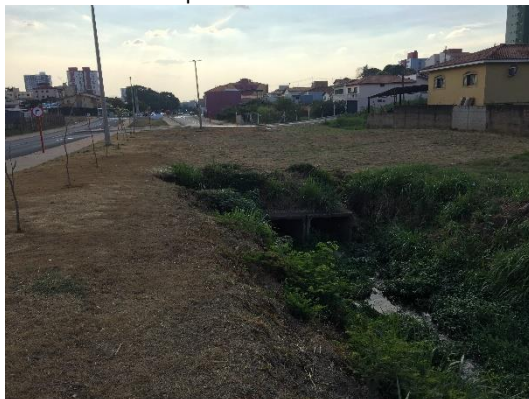
Point 7b - Beginning of buried stream section seen from upstream to downstream
