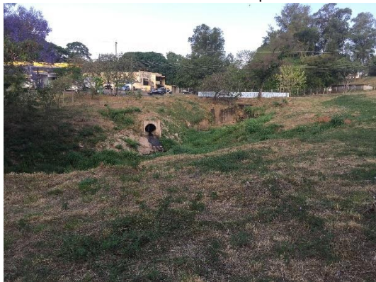
Point 4 - Landslide and pollution focus on the stream seen from downstream to upstream
