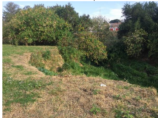
Point 5 - Landslide in the stream seen from downstream to upstream
