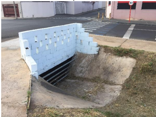
Point 8a - Drainage structure in the buried stream section seen from upstream to downstream
