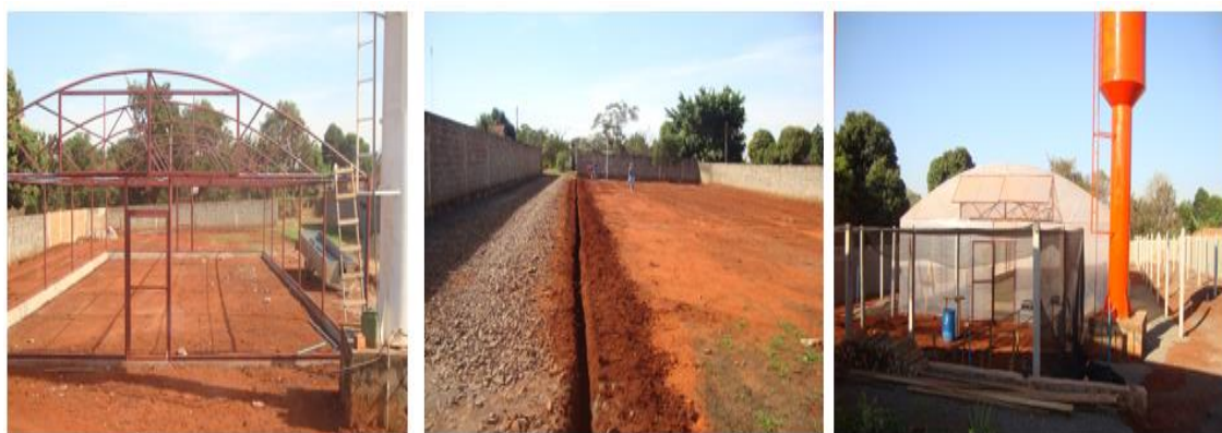
Figure 2 - Images of the construction phases of the Municipal Nursery “Flora do Cerrado”, Campo Grande, Mato Grosso do Sul
