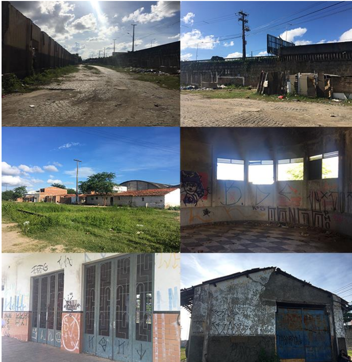
Figure 6 – Current situation of the buildings and surroundings at the New Railway Station.
