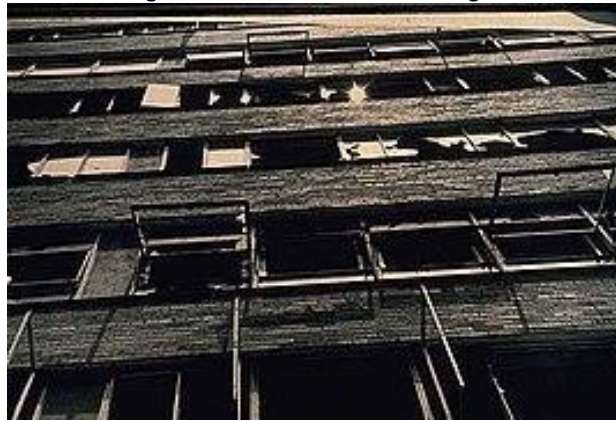
Figure 2 – Deterioration of Pruitt-Igoe
