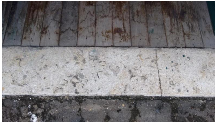
Figure 5: Marble door frame of the Chapel. Note the wear on the floor due to the rain.
