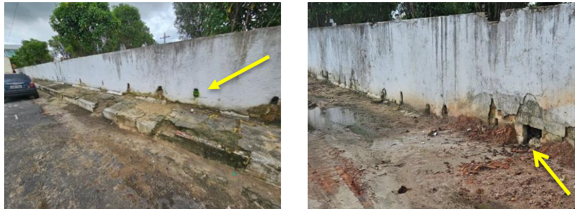
Figure 6. Overflows for surface water drainage in the Santa Rosa de Lima cemetery, Bragança, Pará.
