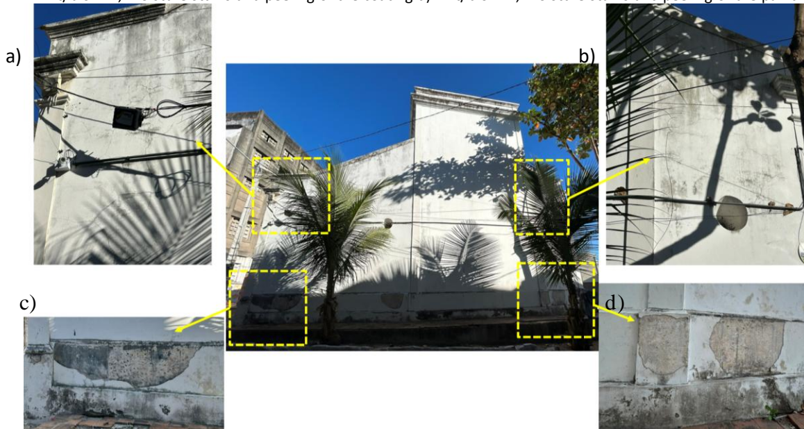
Figure 5 – Pathological manifestations of the North Facade: a) Dirt/biofilm, cracks b) Dirt/biofilm, cracks c) Dirt/biofilm, moisture stains and peeling of the coating d) Dirt/biofilm, moisture stains and peeling of the paint
