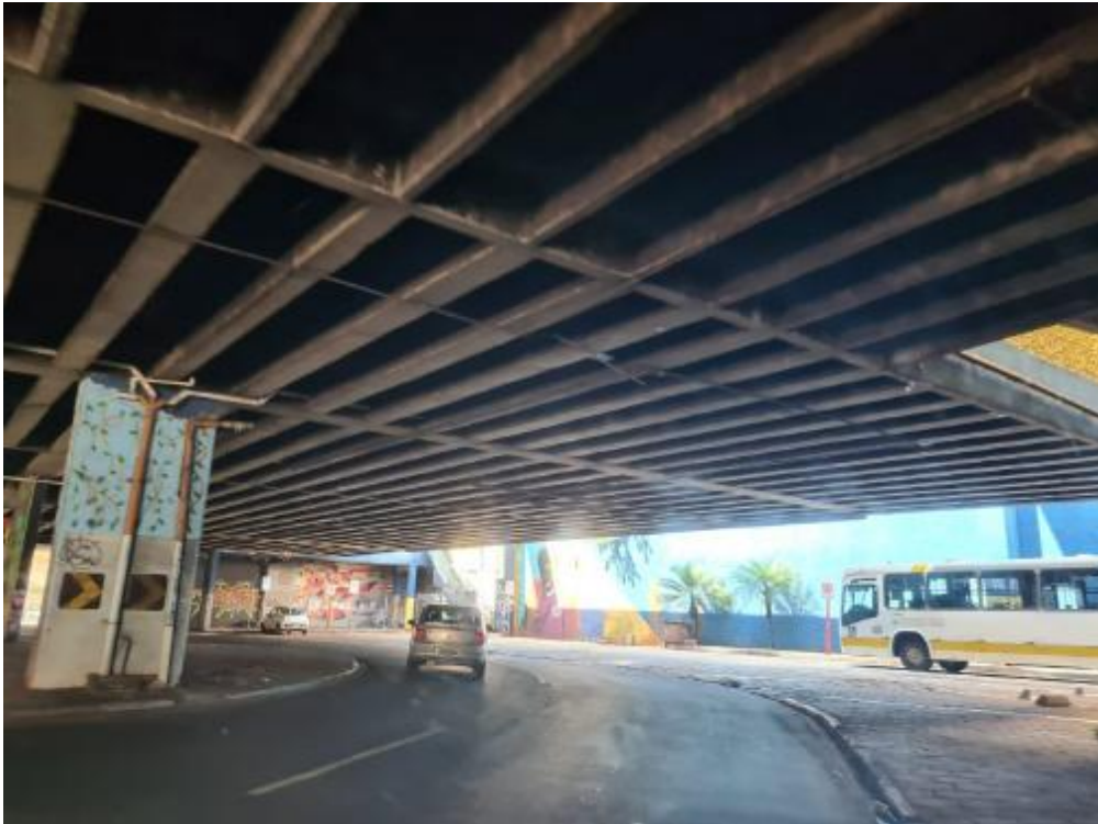
Figure 5 – Area below the Terminal where flooding occurs
